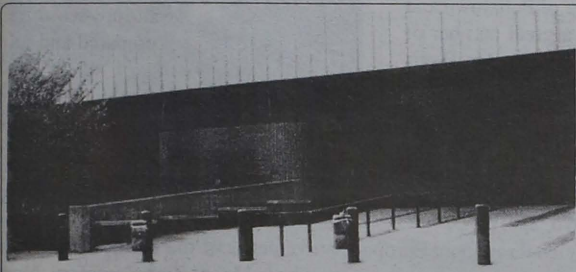
Danger! Danger! Students have been advised to stay clear of the basement area in Helfferich Gymnasium due to the recent asbestos outbreak. Staff Photo by Stephanie Restine
