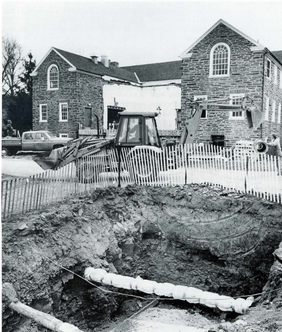
The back of the old union building was demolished to make way for a new main entrance and provide for additional public and utility space inside.
